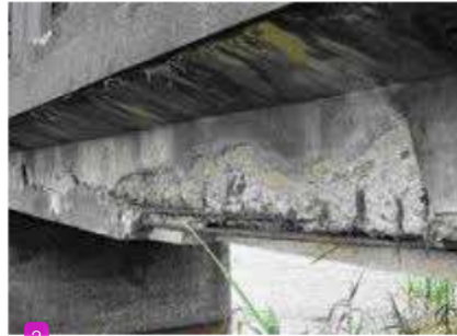
Figure 1. Damage to concrete structures due to corrosion.
